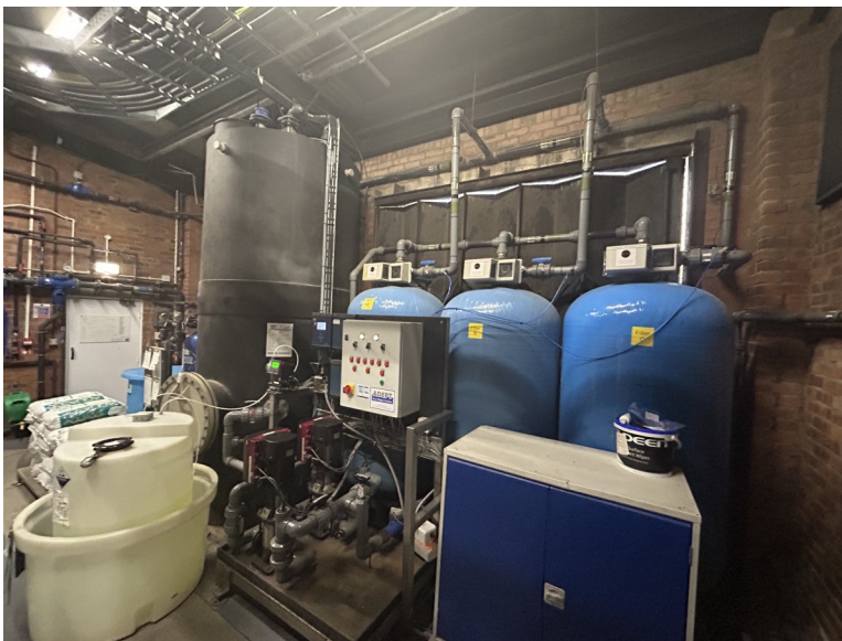
Figure 5: Whitby Seafoods plant room.
