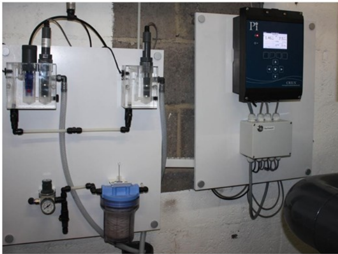
Fig.3 - A picture of one of the CRIUS® controllers installed at Crow Wood Leisure
